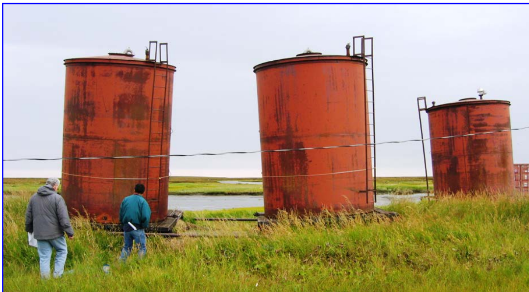
Aging and deteriorating fuel tanks
